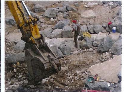
A spotter works with the machine operator to ensure proper stone fit (above).
